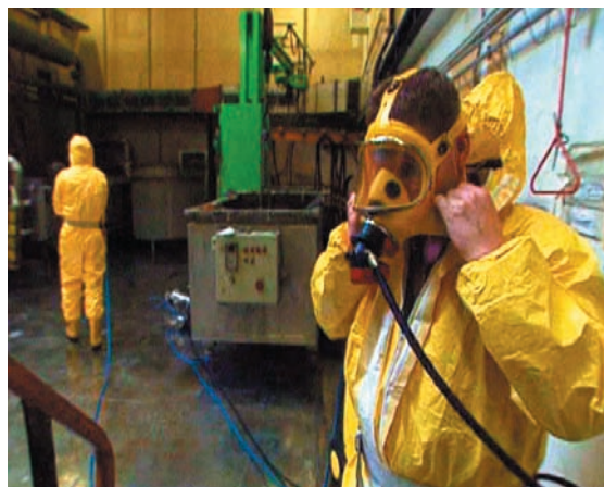
Greifswald NPP (Germany). The personnel prepares for dismantling of the radioactively contaminated equipment
