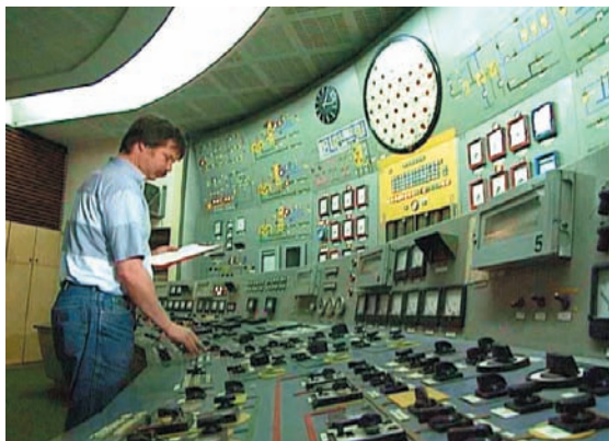
Control room of the Greifswald NPP
