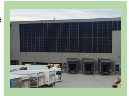
Warehouse in Lier with solar panels
